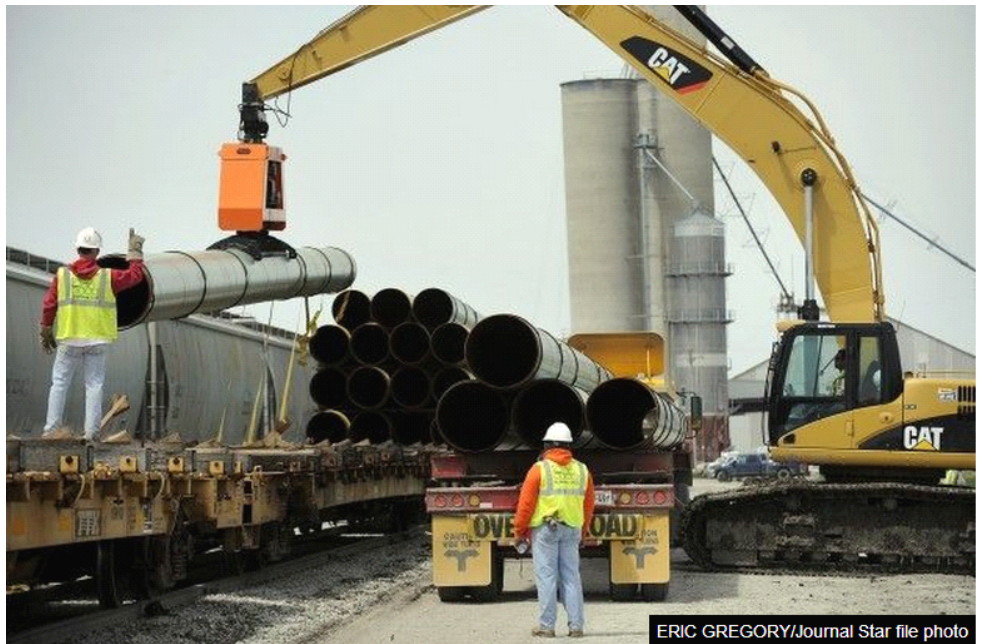
A crew offloads 10,000-pound sections of pipe from a railcar just east of David City in 2009 during construction of the first Keystone pipeline. A look at retail sales tax receipts during the pipeline's prime construction year shows little evidence of a consistent economic boost.
